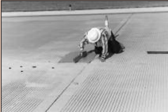
Product: Transpo's T-17 Rapid Patch Project: Airfield Pavement Rehab, CIP #4910-8107-3081, CIP ID# 6000-028 Location: Bergstrom International Airport, Austin TX Size: 5-7,000 Square Feet, Min. 2.5" Deep Engineers: URS Corporation/CH2MHill, Austin TX Contractor: EAS Construction LP, El Paso TX Project Manager: Bobby McClelland
