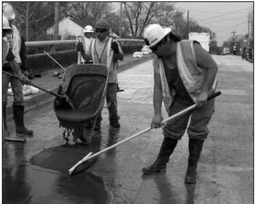
Material: Transpo's T-48 Slurry Location: Chickasaw Bridge, TN Contract: Project #19960-4216-04 Size: 26,000 Square Feet Application Time: 12 Hours Owner: Tennessee DOT Contractor: Jamieson Construction Supplier: Hiwassee Materials, Charleston TN, John M. Simpson, P.E.
