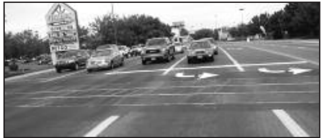
LED Warning Lights built-in to the edge beams at this railroad crossing
